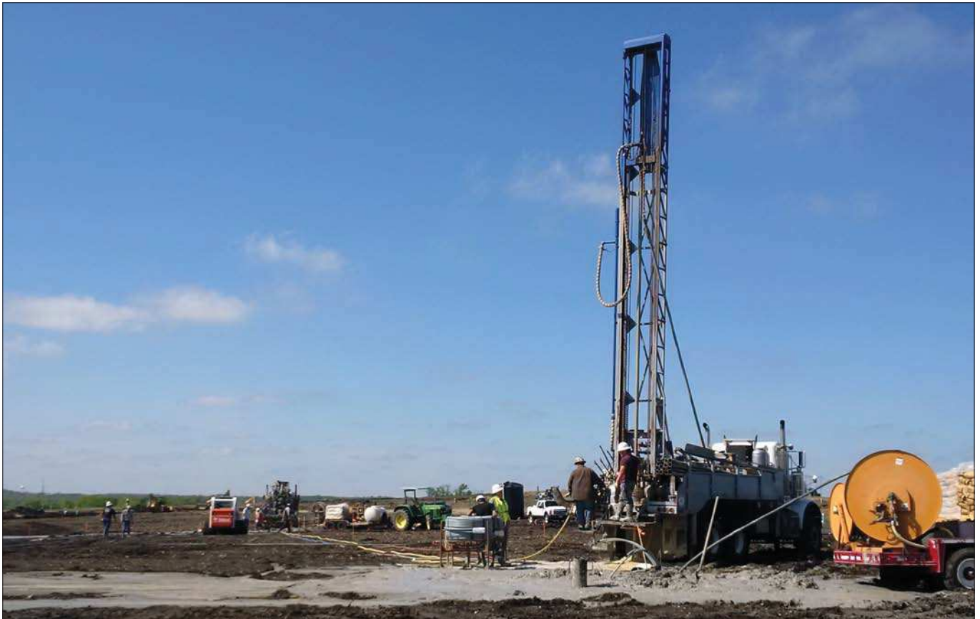
Geothermal energy for a whole urban district? In Whisper Valley in Austin/Texas the first drilling works are taking place.
